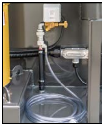
Automatic Water Fill with Soap Injector
